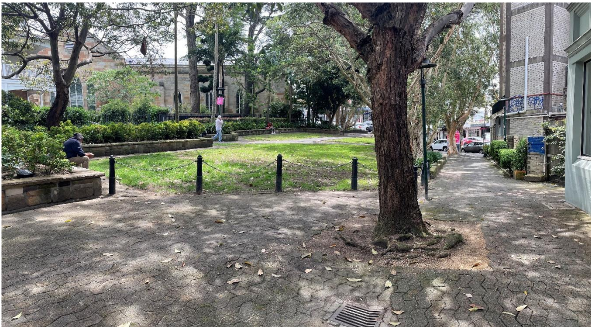
Looking north towards Oxford Street from Regent Street. Uneven paving caused by the trees. Bollards stopping unwanted movement on to grass. End of life lighting and stormwater visible.
